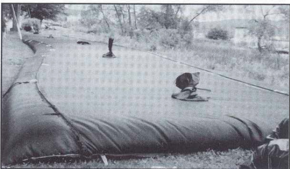
After sitting overnight, the bag is dry. The volume of material can shrink as much as 70 percent, so material can be pumped into the bags many times before they are filled.
