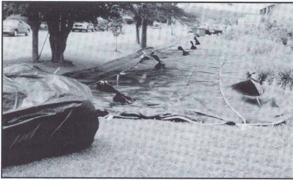
The first bag has been rolled out on the old railroad right of way. Fill ports are visible along the top, tied off when not in use.
